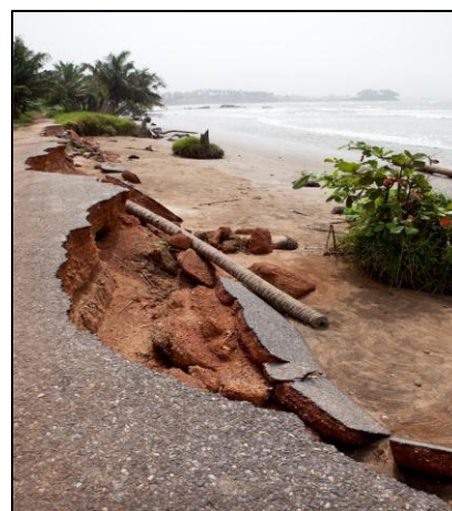
Figure 2: Washed feeder road along Ankobra beach
